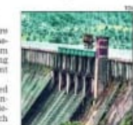
The leakage was spotted by several locals who then informed the irrigation department
